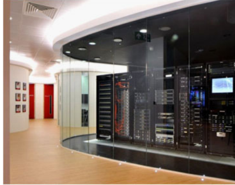
Figure 4. Server room, on-premises data storage. Source: pinterest
