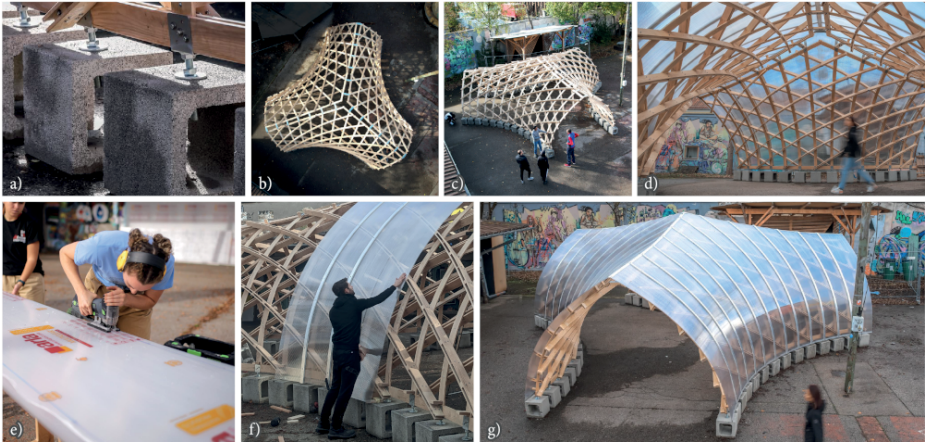
Fig. 8: Completed timber gridshell. Top Row: a) Precast concrete blocks with steel supports. b,c) Birds-eye view of the timber gridshell without cover. d) Inside the Timber Vault. Bottom Row: Polycarbonate panels are tailored with concave edge (e), and installed using aluminum mullions along the geodesic directions (f), to create a smooth, transparent skin (g).
