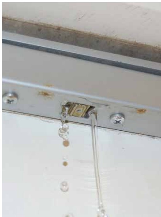
Fig. 4. Water entering the building because of inadequate flashing.
