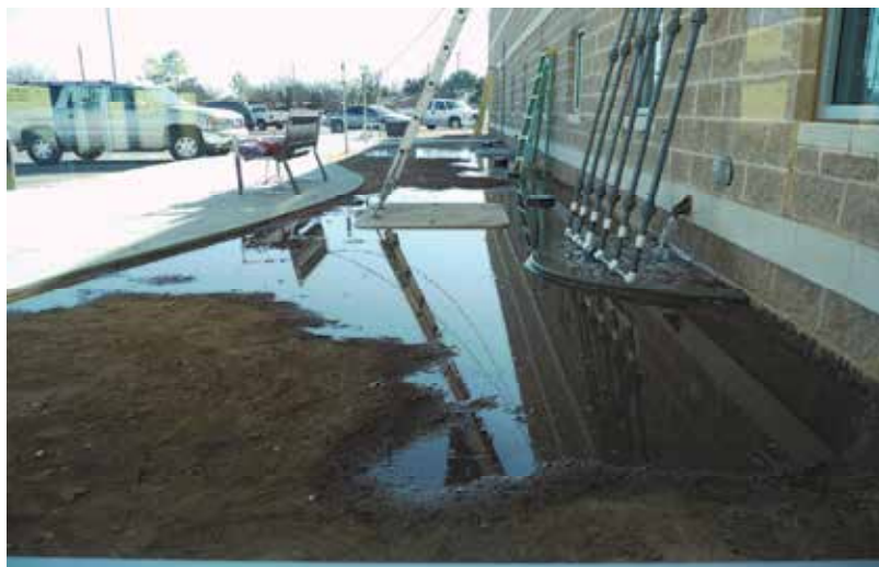
Fig. 11. Improper site grading.
