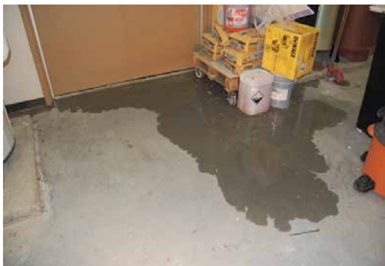
Fig. 7. A flawed detail at the base of the building compounded the threat to the building posed by standing water.
