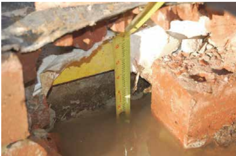
Fig. 9. Water standing inside the wall cavity.
