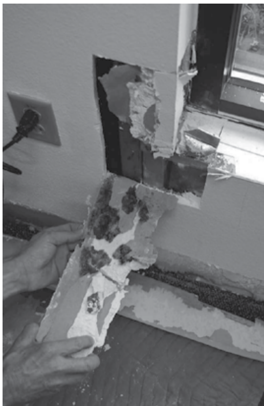
Fig. 3. Mold caused by moisture in the wall cavity.
