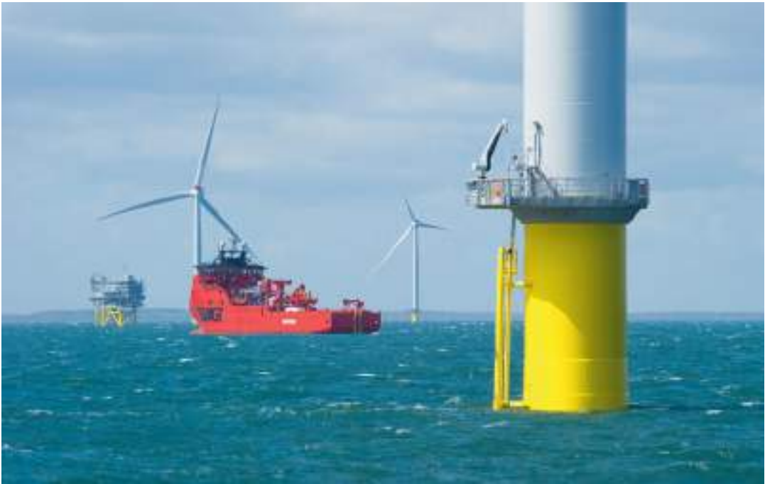
Fig. 26.2 The Westernmost Rough offshore wind farm under construction, located 8 km offshore of the Yorkshire coast near the Humber estuary, giving some idea of the infrastructure involved in wind farm installations. The total array covers an area of 32 km 2 with 35 turbines, three of which are visible in this photograph, connected by 53 km of submarine cables, and an offshore electricity substation, visible on the far left. The red ship is a specialist vessel for servicing the turbines. © Historic England Archive, Alun Bull
