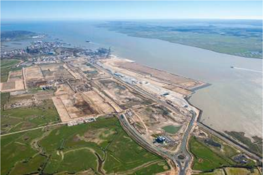
Fig. 26.1 Construction work in progress at the London Gateway Port development on the Essex coast in the Thames Estuary, giving an impression of the area affected and the potential impact on the historic environment. © Historic England Archive, Damian Grady
