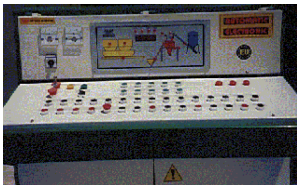
Fig. 12. The central board of plant control and monitoring
