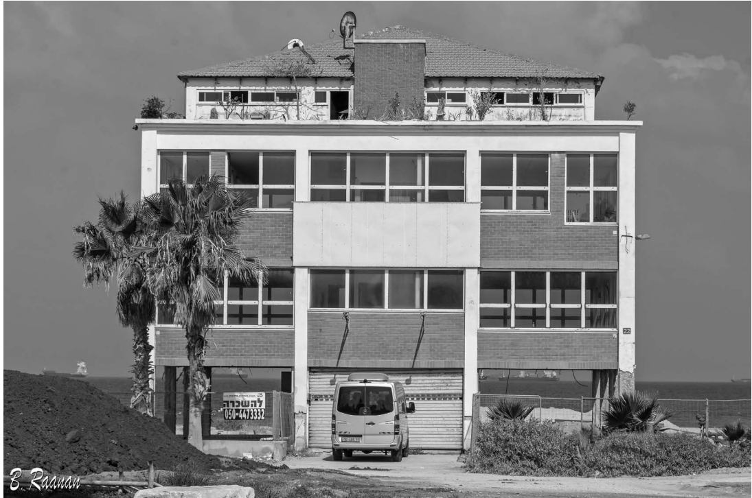
Figure 15.6 Illegal “kiosk” extension at Lido Beach, Ashdod (before partial demolition)
