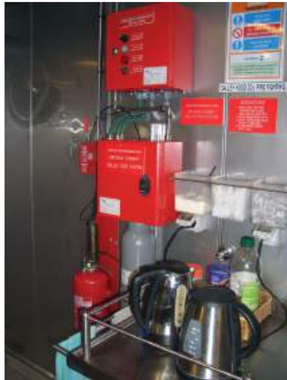
Plate 211 CO 2 / inert gas supply and control to galley hood.
