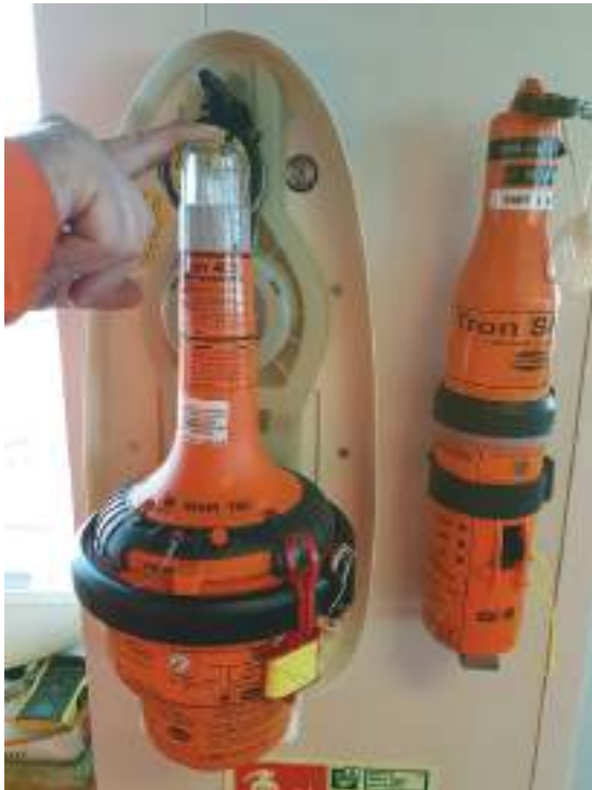
Plate 122 Example EPIRB, emergency position indicating radio beacon bulkhead mounted alongside a SART.
