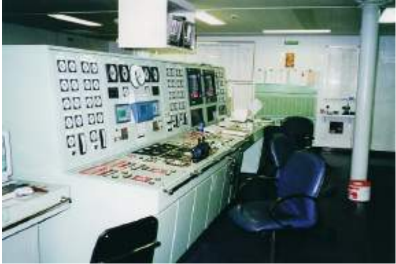
Plate 224 Main engine control room for modern twin-screw passenger ferry.
