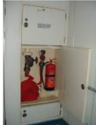
Plate 208 Hose box station inside the accommodation of a large passenger vessel. Contents include hose pipe and nozzle connected to hydrant, portable 9 ltr fire extinguisher and a wheel key for valve operation. A sprinkler section test station is enclosed.
