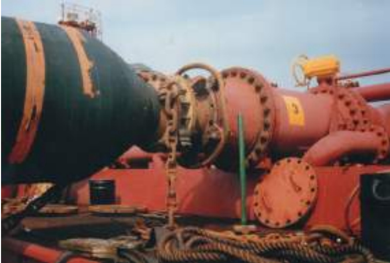
Plate 269 Pipeline/manifold connection aboard a large tanker vessel.
