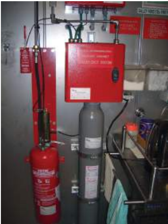
Plate 210 Inert gas arrangement fitted inside a pantry next to the galley. Operates to flood galley air ducts.
