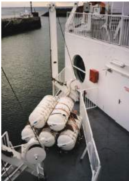
Plate 95 Rack stowage of davit-launched inflatable life rafts aboard a passenger vehicle ferry.
