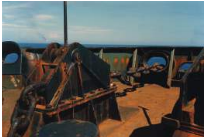
Plate 263 Chafe chain moorings secured with AKD stoppers aboard a tanker vessel engaged in oil transfer from floating storage unit (FSU).
