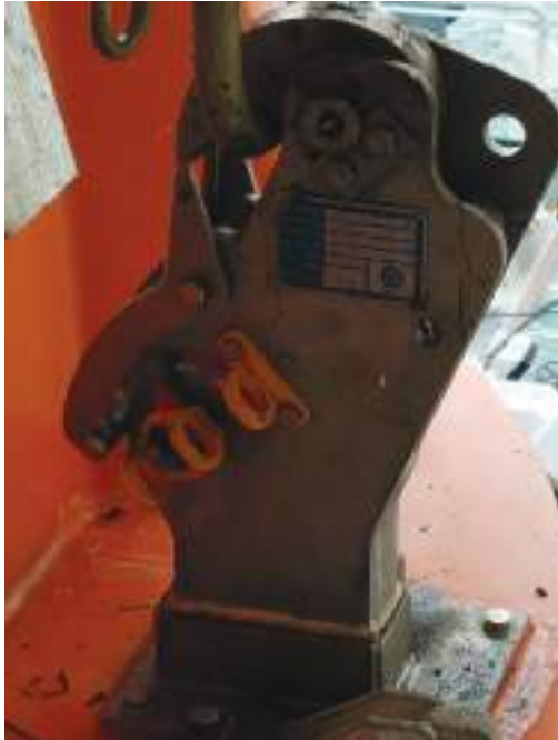
Plate 91 Fall preventative at locking pin removed allows the fall hook to trip.
