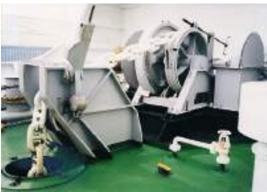
Plate 15 Arrangement of the starboard windlass aboard a modern ro-pax ferry with split windlass operation. The guillotine bar, bow stopper, is seen in the open vertical position.
