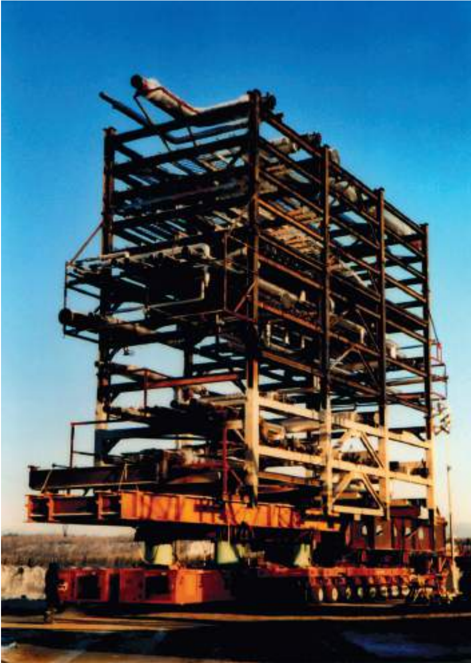
Plate 38 Multi-wheel road transporter moving an offshore installation section prior to loading to a sea transport towards a cold platform under construction.
