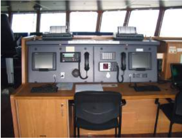
Plate 119 GMDSS communication console seen aboard a new ro-ro ferry vessel, operating out of the United Kingdom. (Source: Capt. David A. McNamee AFNI.)
