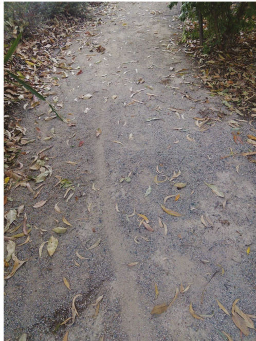
Figure 5. Loose gravel path.
