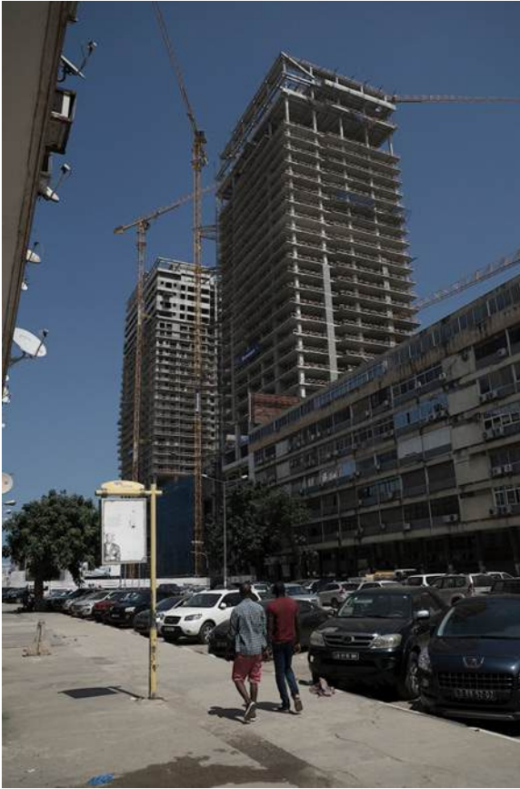
Figure 4.1. View of Kinaxixe Square in 2015 after the destruction of Kinaxixe Marketplace. Source: Rui Sérgio Afonso.
