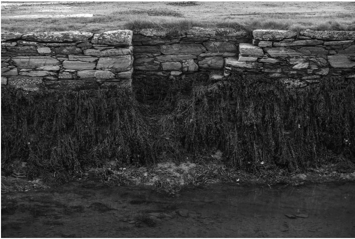
Figure 7.6 A detail of the Quay wall showing pinnings and traces of lime mortar. Photograph by Kevin O'Farrell 2021.
