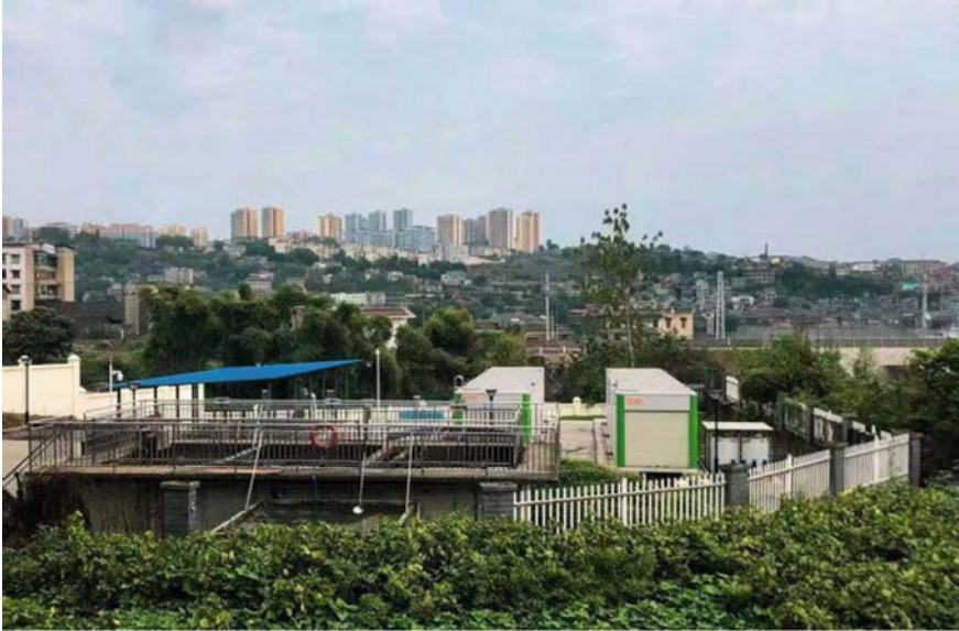
Fig. 5.14 The site of a rural domestic sewage treatment case in Chongqing Yangtze River protection spots
