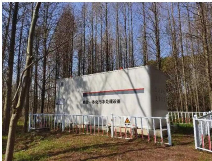
Fig. 5.10 The site of a rural domestic sewage discharge standard upgrading case in Chongming District, Shanghai, China
