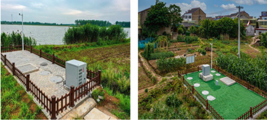
Fig. 5.8 The site of a rural domestic sewage treatment case in Liuhe district, Nanjing, China
