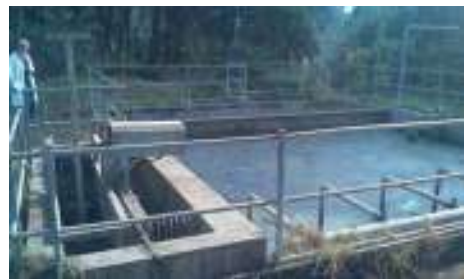
Defective sewage treatment plant in September 2013
