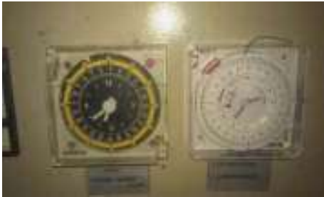
The sewage treatment plant was put back into operation after a new timer was installed
