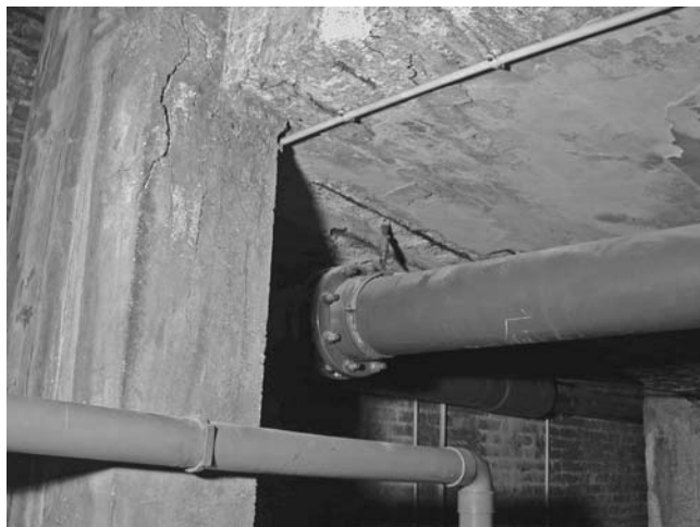
Figure 2.11 Degradation of concrete in the technical area underneath a swimming pool.
