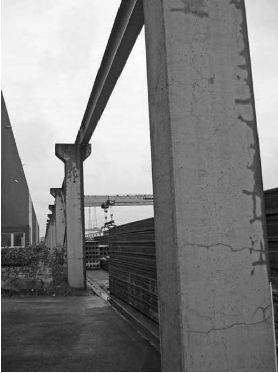
Figure 5.27 ASR in concrete columns.
