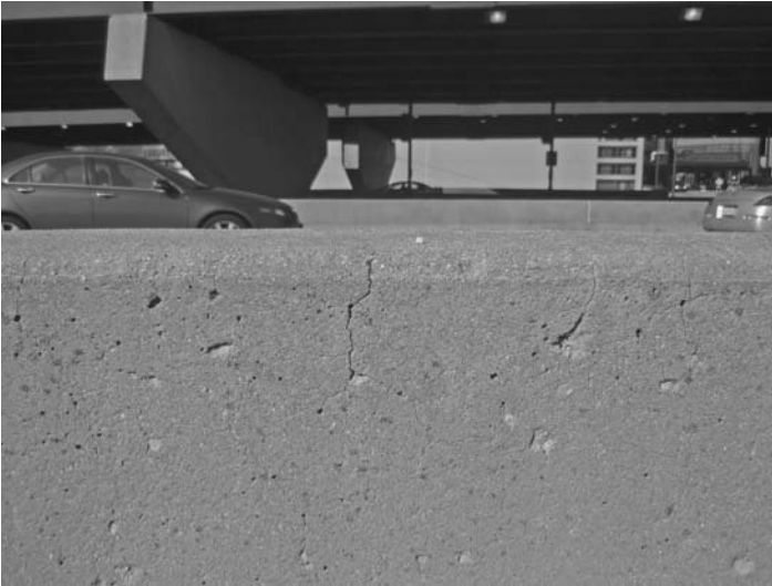
Figure 4.6 Drying shrinkage cracking in New Jersey concrete barriers.
