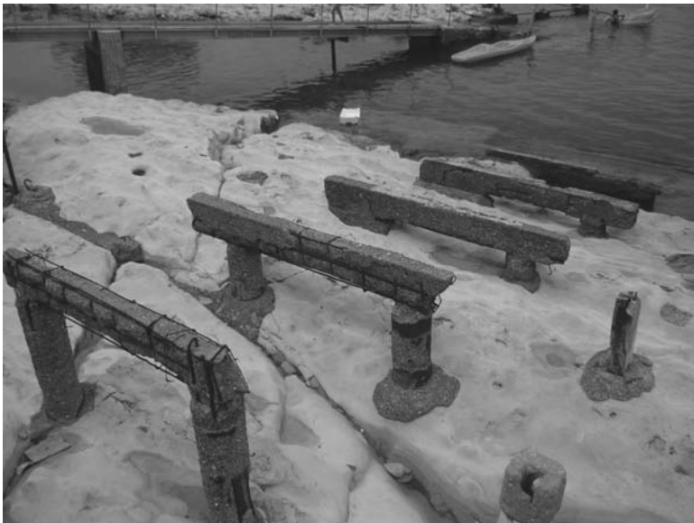
Figure 5.47 Chloride induced reinforcement corrosion in some concrete elements near the Adriatic Sea.
