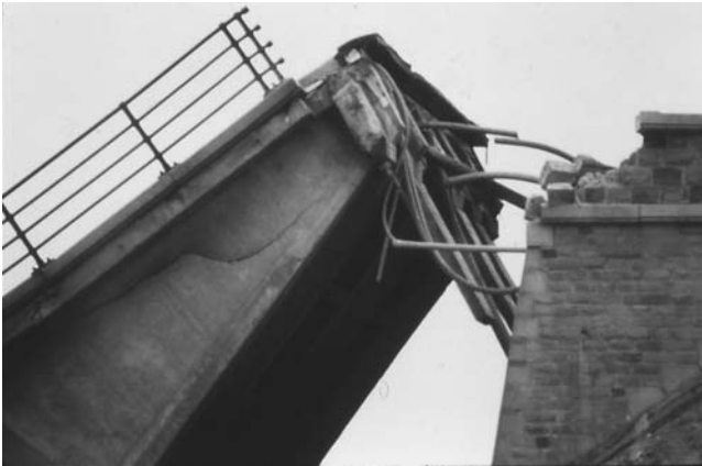
Figure 2.3 Picture of the tensile pendulum pillars (after failure).
