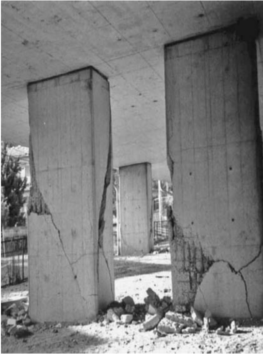
Figure 5.2 Damage to concrete columns due to earthquake loading (Internet photo).
