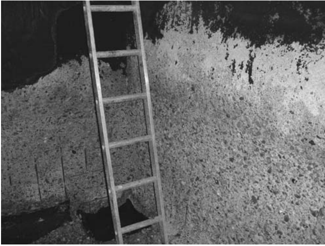
Figure 5.34 Sulfuric acid attack on a concrete wastewater tank in an industrial plant (courtesy of SCICON Worldwide bvba).
