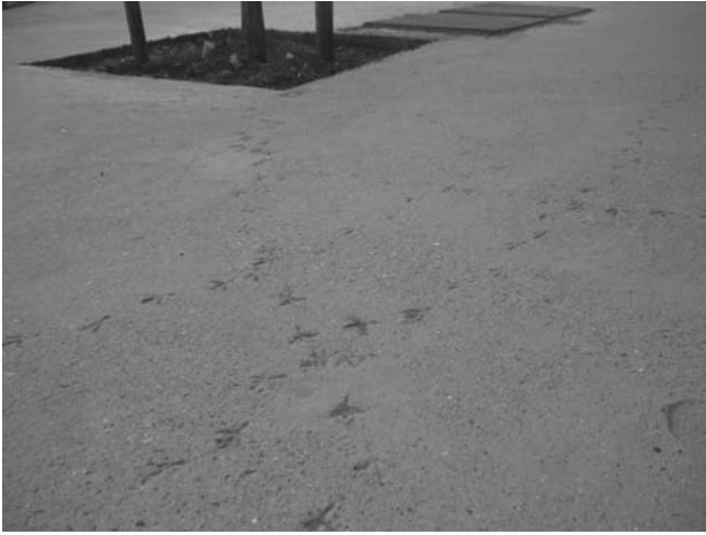
Figure 3.15 Damage by animals walking in freshly cast concrete.
