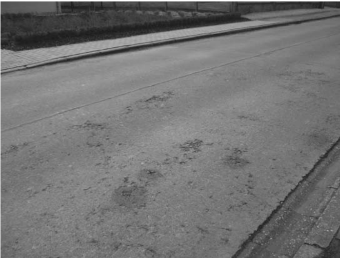
Figure 5.12 Salt scaling on a concrete road.
