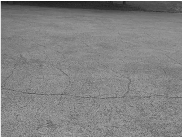
Figure 3.18 Parallel plastic-shrinkage cracks (wind cracks).
