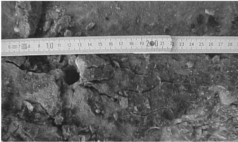
Figure 5.30 Detail of a concrete balcony damaged by expansive chemical sulfate attack (courtesy of SCICON Worldwide bvba).
