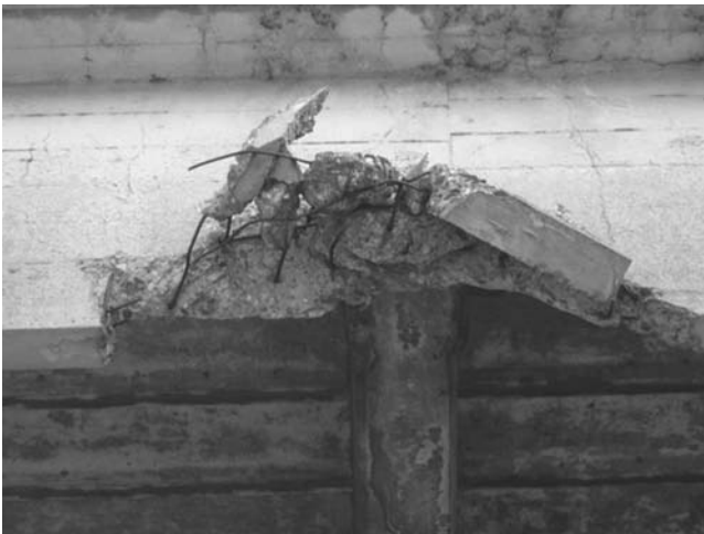
Figure 5.3 Impact damage to concrete girder by truck.
