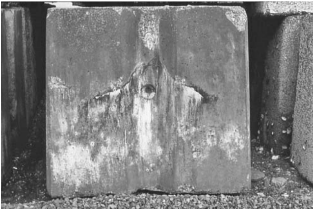
Figure 4.10 Early-age thermal cracks in grooved cube concrete armour unit.
