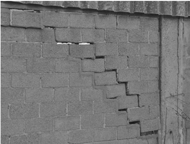
Figure 5.6 Effect of differential settlements on a concrete brick wall.
