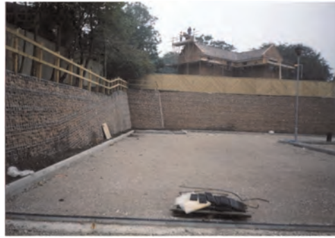
Figure 6. Gabion stone faced wall nailed on left boundary full RSS on adjacent face 1998 (Comtec UK Ltd).
