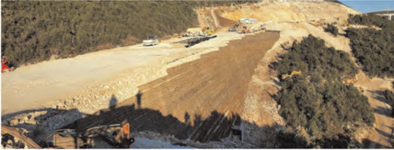
Figure 4. Replacement of the Doli viaduct with a wrap-around geogrid reinforced embankment (span 180 m, maximum height over 17 m).
