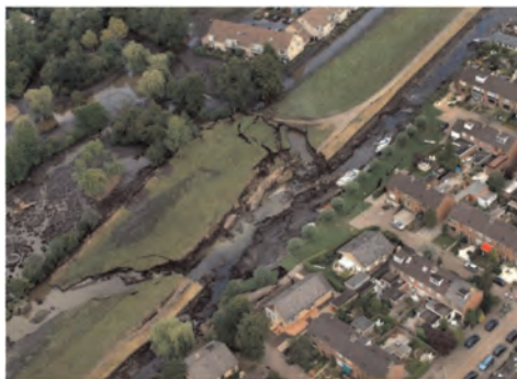
Figure 3. Aerial picture peat levee collapse, caused by dehydration during extreme drought, 2003 Wilnis Netherlands.
