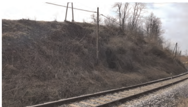
Figure 1. Unstable slope near railway line in Mirna Peč (Slovenia).
