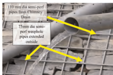
Figure 13. Sub-surface water discharge through weepholes.
