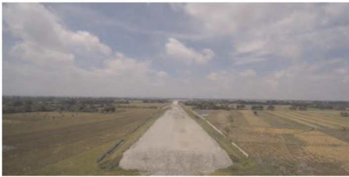
Figure 4. Placement of drainage sand blanket layer prior to placement of geotextile reinforcements.
