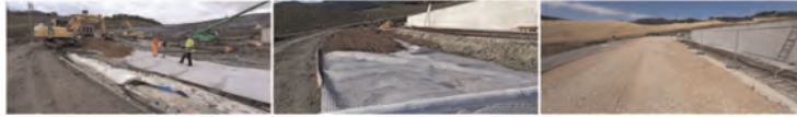
Figure 5. Construction phases of internal roads with the use of base geocomposite reinforcement.
