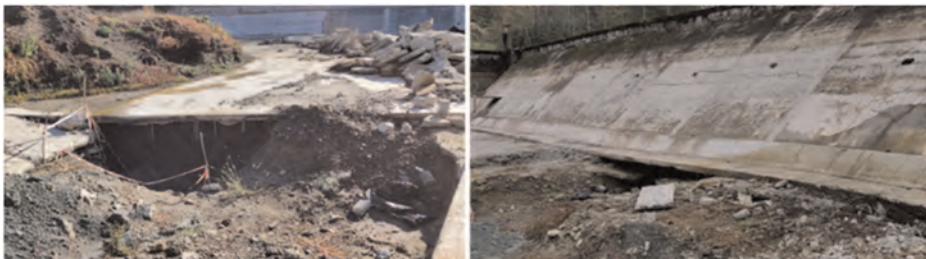
Figure 5. Pictures of the 2020 failure.
