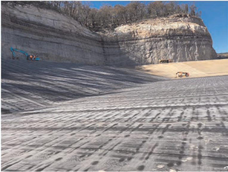
Figure 3. BGM being used for environmental protection by containing stormwater run off from a mine before it reaches the river. New South Wales, Australia.
