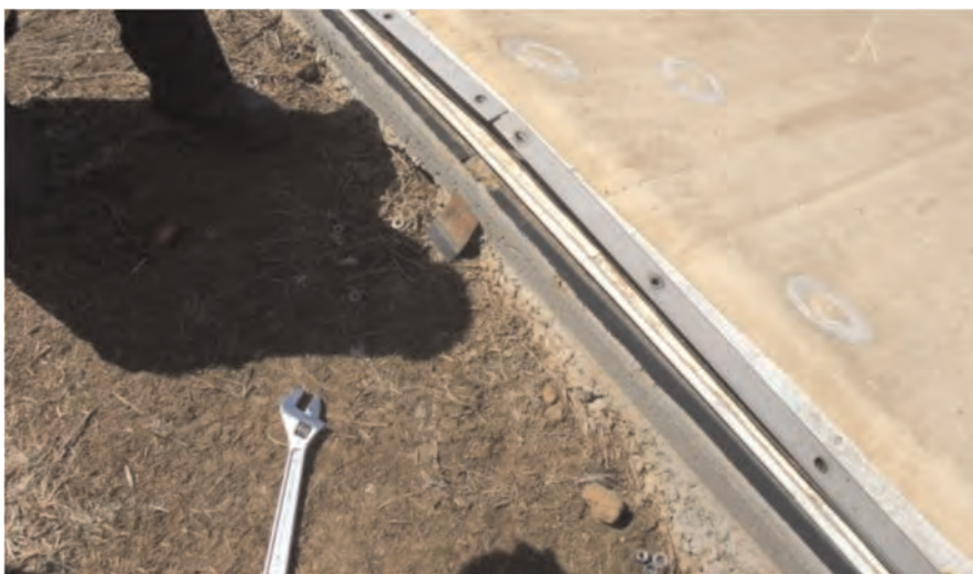
Figure 2. A small liner material sample taken from under a batten bar. This floating cover had many small marked holes which had been caused by embers from a grass fire.
