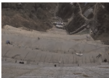
Figure 10. Berm provided to collect & drain surface water.
