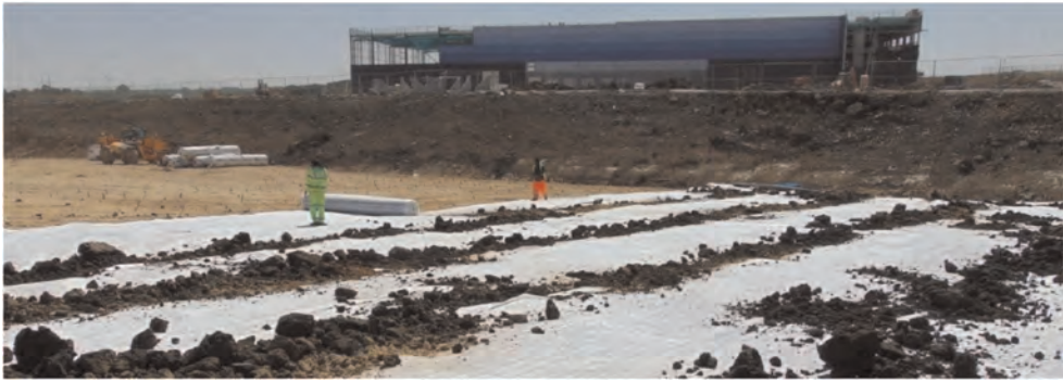
Figure 6. Placement of starter layer geocomposite prior to raising of formation level (ABG Geosynthetics Ltd).
