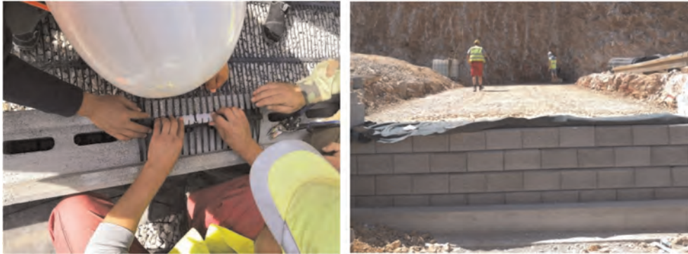
Figure 2. a) Top view of the concrete blocks with the connectors and the uniaxial extruded geogrids; b) Front view of the first row of blocks placed against the tooth of the concrete foundation pad.
