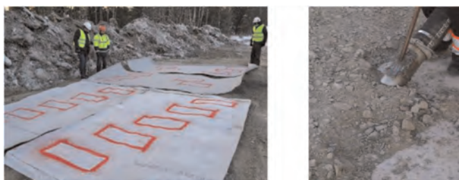
Figure 5. Installed geosynthetic samples with drainage function and recovery of the drainage composites.
