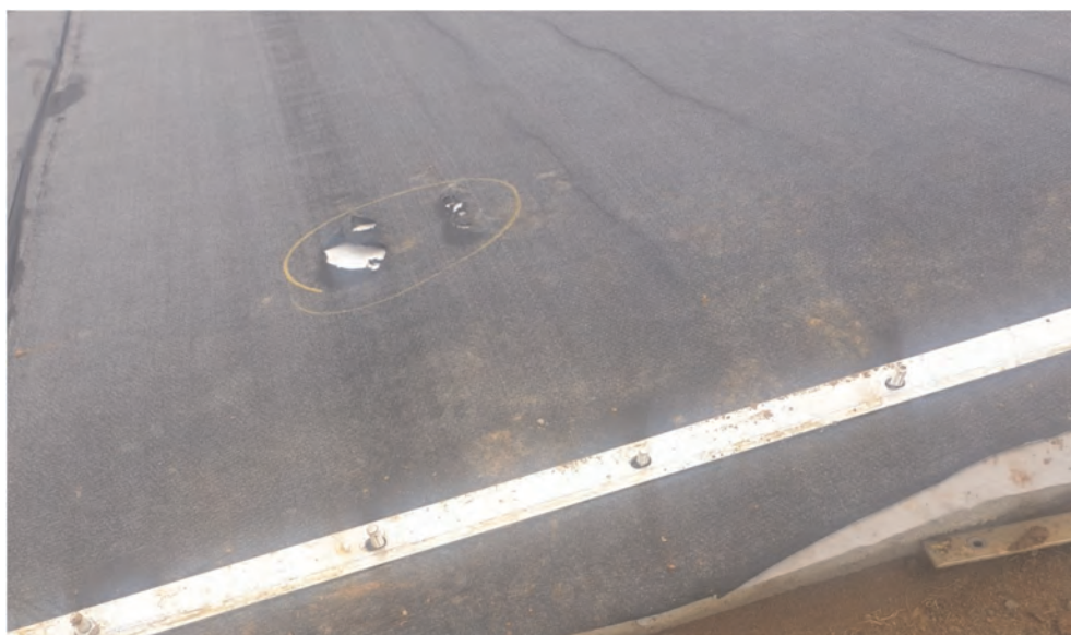
Figure 5. Holes in a conductive composite made by workers walking on it. These required patching to ensure adequate conductivity.
