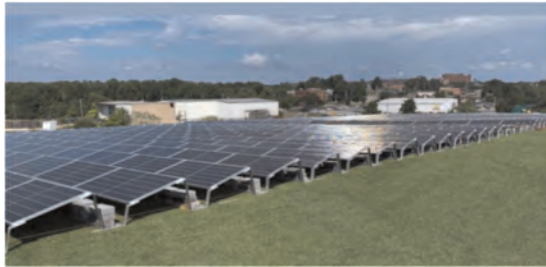
Figure 6. Community Solar farm installed on engineered turf cover at the Cranston Sanitary landfill, Cranston, RI.
