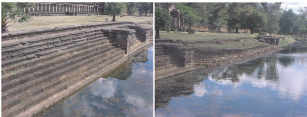
Figure 2. Adjacent portions of the steps showed a different behavior due to different boundary conditions. Left: dry assemblage of the steps; Right: Joint sealing (gray cementitious mortar) preventing drainage.
