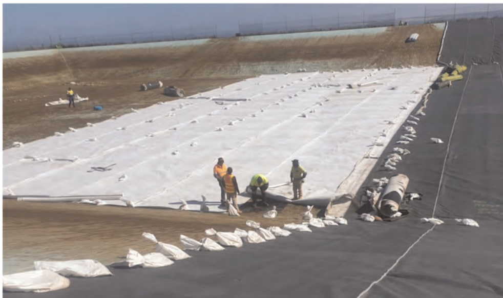
Figure 3. A reservoir with the old discoloured fPP liner being used as a secondary liner. The white material on the floor is a drainage geocomposite and the black material on the slopes and the floor is a conductive non-woven geotextile with a unit mass of about 350 gsm.
