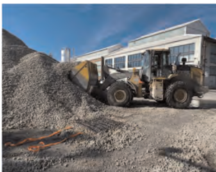
Figure 1. Photograph of UL-FGA installation.
