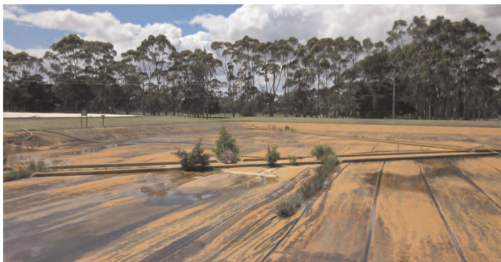
Figure 7. A 30 year old CSPE cover where a lack of maintenance has allowed vegetation to grow.
