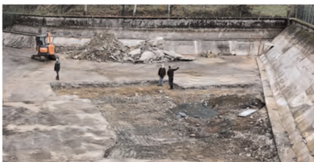
Figure 6. Internal erosion of foundation under the removed damaged slabs.
