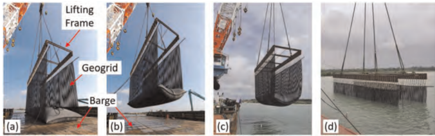
Figure 7. Lifting and lowering process: (a) Setup of lifting frame and geogrid; (b) Lifting of geotextile tube from the barge; (c) Shifting of barge that was used to install the geotextile tube; (d) Lowering of Geotextile tube into the water.
