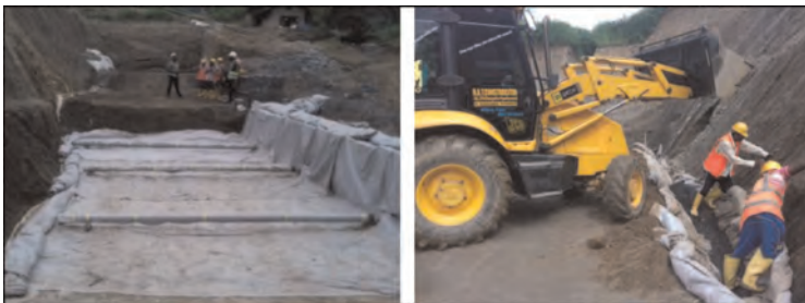
Figure 6. Placement of drainage pipe (left) and drainage blanket at the back of the slope (right).
