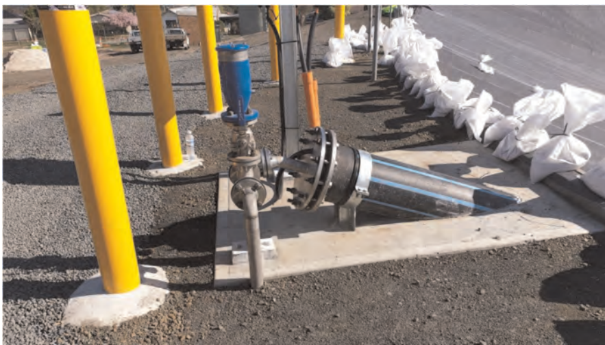
Figure 4. An underdrain water extraction system with a down the slope pipe with a bore pump.
