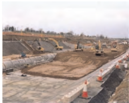
Figure 8b. Membrane over central collector.
