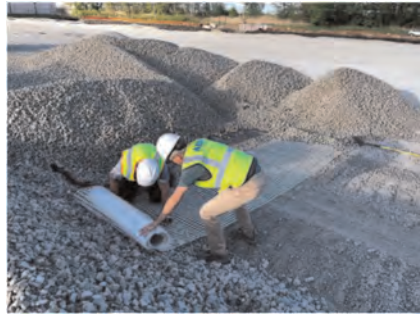
Figure 6. Photograph of PHL Ron installation.
