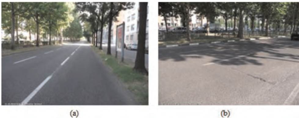
Figure 2. HaTelit C 40/17 reinforced area without cracks (a) and unreinforced section presenting reflective cracking (b) (July 2009).
