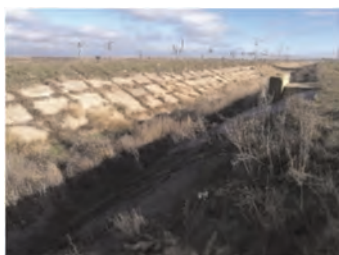
Figure 6. concrete for canals some years after due to unstable soil underneath.
