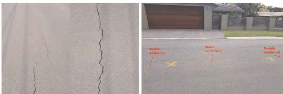
Figure 6. Performance of unreinforced (left photo) vs single reinforced and double reinforced sections (right photo) on expansive subgrade.
