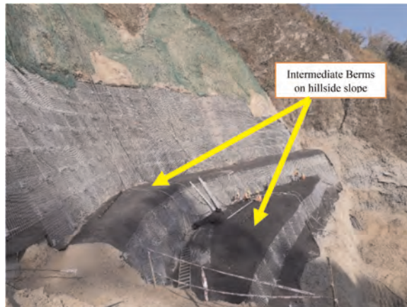
Figure 14. Slope stabilization through installation of soil nails and fixing one layer each of non-woven geotextile and GI back mesh.
