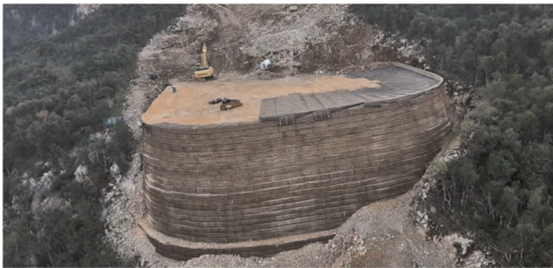
Figure 8. Front drone view of the U4 wing wall and abutment of the Dumanja Jaruga viaduct constructed using a wrap-around reinforced soil technique with a sacrificial steel mesh formwork at the face and mono-oriented extruded geogrids in HDPE.
