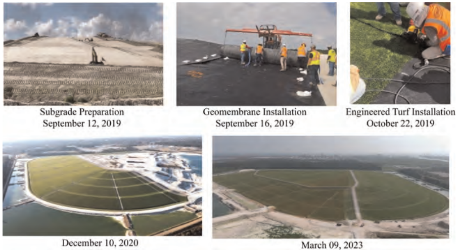
Figure 2. Engineered turf cover construction at the Mississippi phosphates corporation gypsum stack, a US EPA superfund site.
