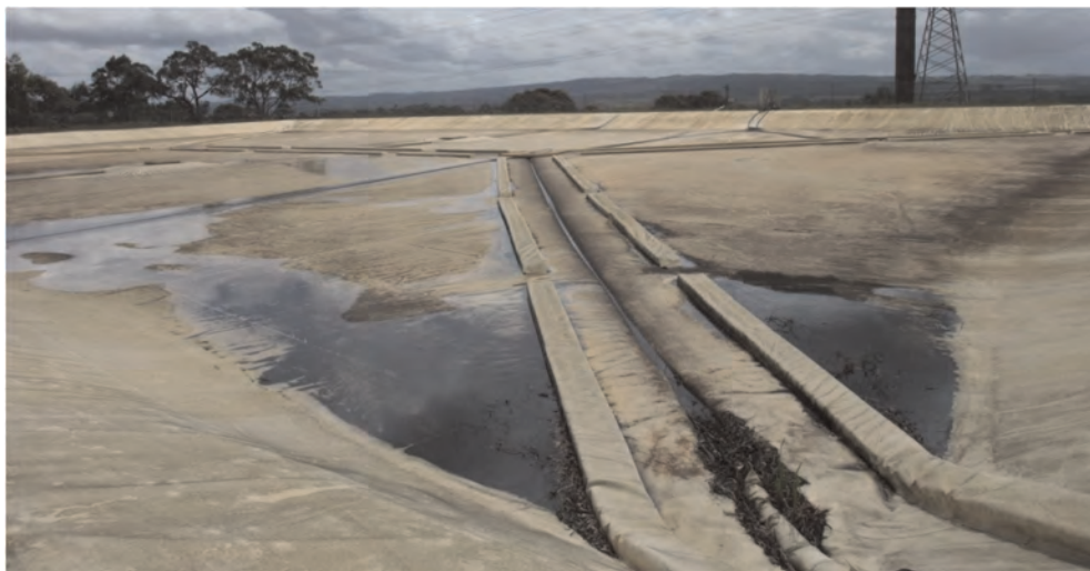
Figure 6. A floating cover with foam floats for tensioning and other floats for access walkways.
