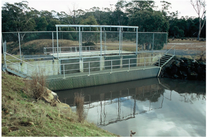
Figure 2. The Lake Crescent outlet structure showing the coarse external screens.
