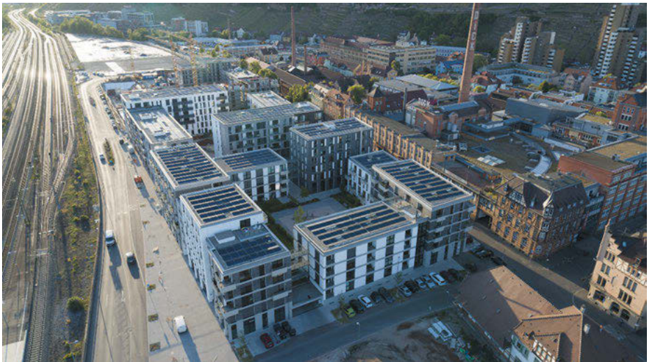
Figure 11.1: Blocks B, C, and D (in construction). (Source: Maximilian Kamps, Agentur Blumberg GmbH)
