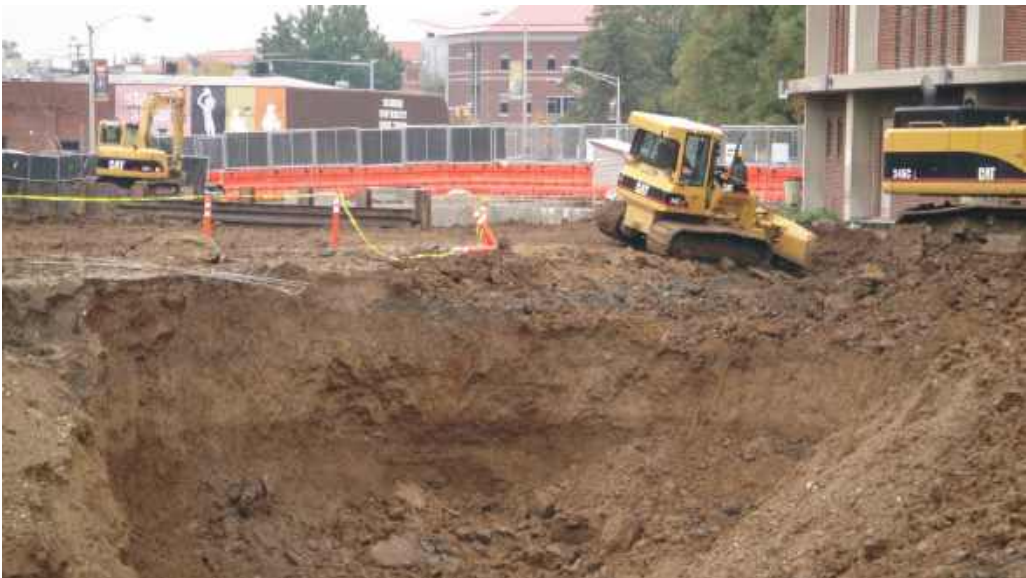
Figure 6-17. Vertical excavation of clay. Despite the initial stability of steep slopes, they must be cut back for safety to at least 0.75H:1V, and maybe more, if a soil retaining structure is not built.
