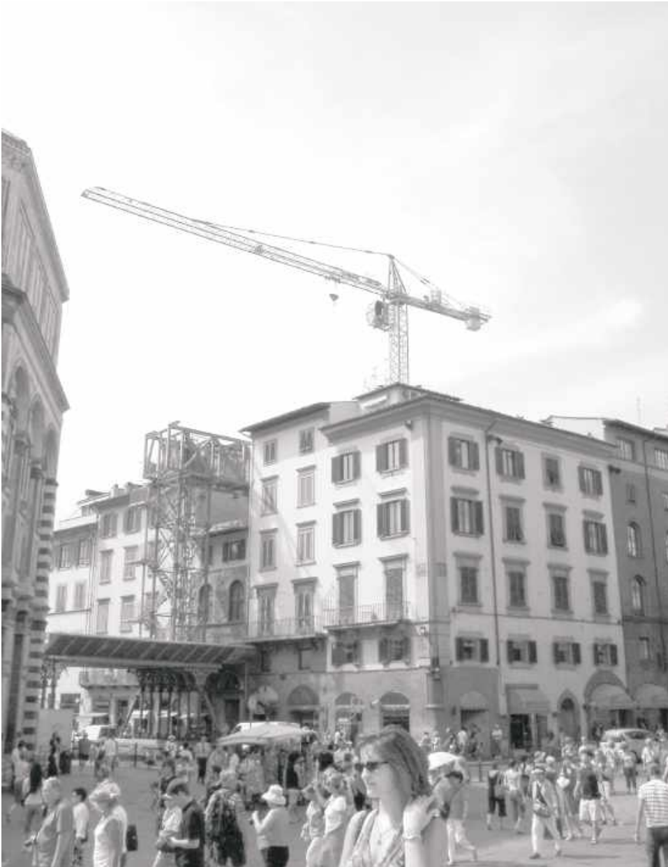
Figure 1-1. Highly restricted work sites adjacent to buildings, as shown in this image from Florence, Italy, can require elaborate and costly scaffolding for access. The planning and permitting for such temporary works are seldom trivial.
