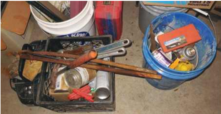
Figure 7-16. Typical example of bad material storage for small projects.
