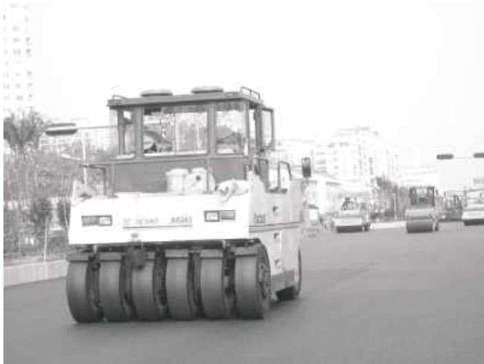
Figure 6-21. Pneumatic-tired roller compacting asphalt. Tire pressure can be regulated to obtain optimum results. This roller type can often be the most flexible for varied compaction requirements.
