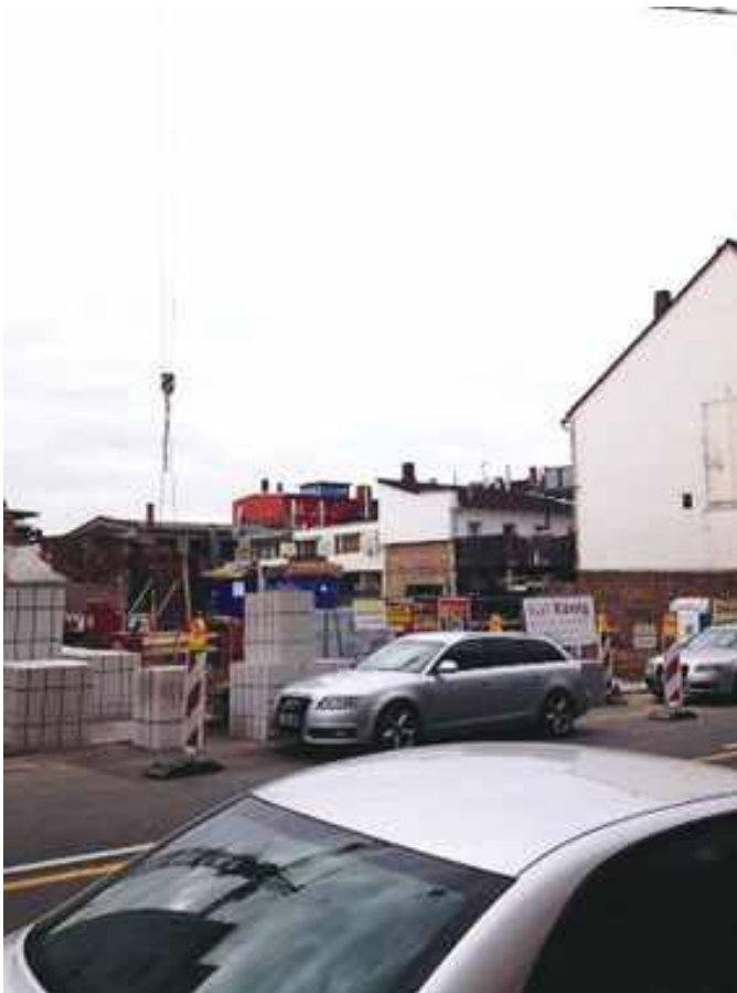
Figure 3-19. Construction site in Darmstadt, Germany, with multiple constraints: restricted site access, no easy locations for deliveries and materials handling, lack of temporary parking, and a clear need for road closures during construction.
