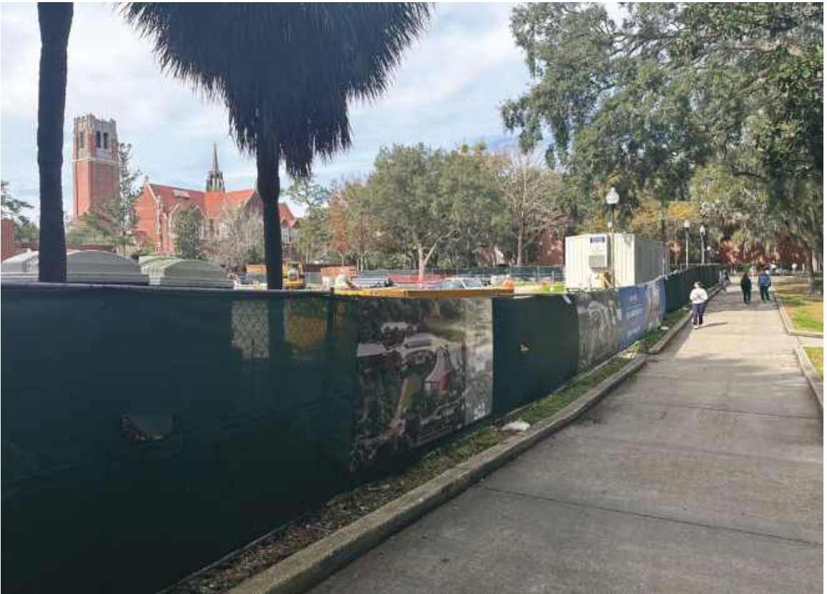
Figure 3-16. Construction activity on the campus of the University of Florida, Gainesville, FL. This walkway must be maintained with full accessibility to ensure the safety and effective flow of faculty, staff, and students through campus (Source: Author, 2024).
