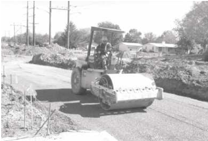
Figure 6-19. Compaction with smooth-wheel vibratory roller. This roller commonly compacts coarse-grained soils and rock fills.
