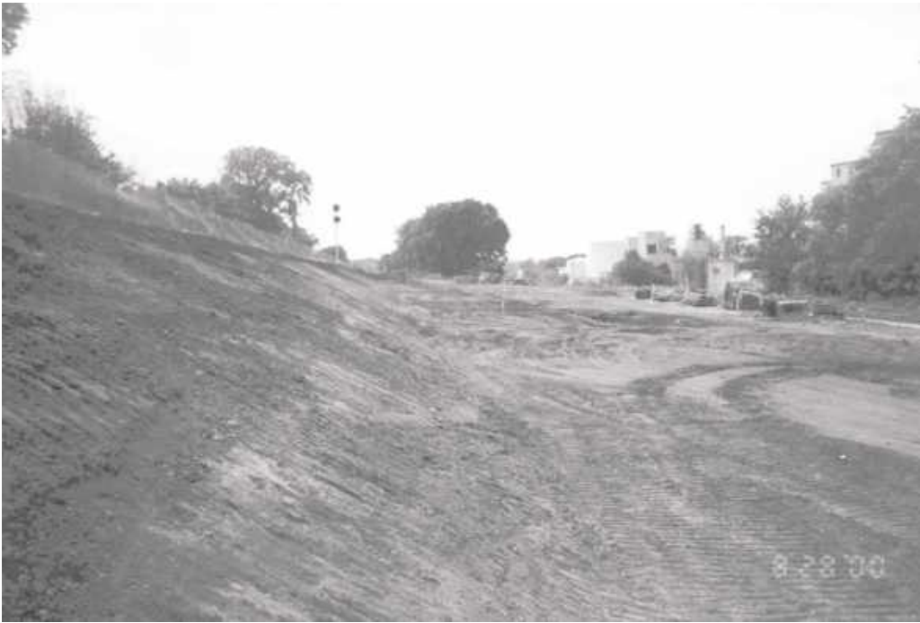
Figure 8-18. The finished product of a mass excavation that employed one track excavator set up to perform mass excavation, several haul units, a dozer designed to grade slopes, a dozer at the dump site (often forgotten in the estimate), and a foreman to manage to process.
