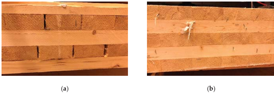
Figure 14. (a) Air gaps in the laminate layers of CLT. (b) No edge-bonding of CLT.
