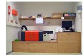
Laser cutters and others are equipped with a filter, like here at Apeldoorn. Caso.
