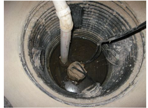
Figure 6.30: A sump crock.
