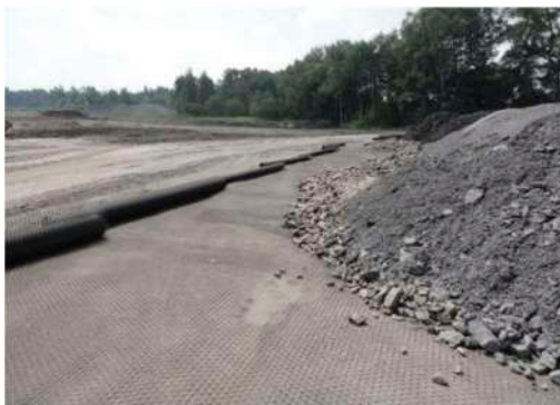
Figure 6. Stabilisation of expressway embankment base constructed from unburnt clay shales – Road 902 project in Gliwice.
