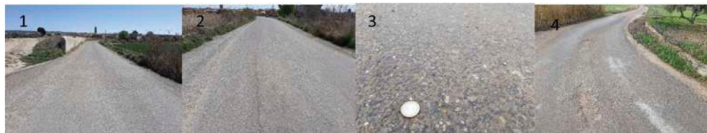
Figure 5. Cement stabilized stretch (1) and WPFA stretch (2) showing a joint. Bituminous treatment integrity (3) and potholes in the joint (4).
