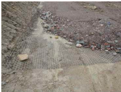
Figure 9. Example of mining waste layer stabilised by geogrid for road construction – road 86 project in Katowice.
