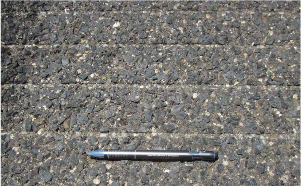
Figure 2. Typical runway surface prior to 2019 resurfacing.
