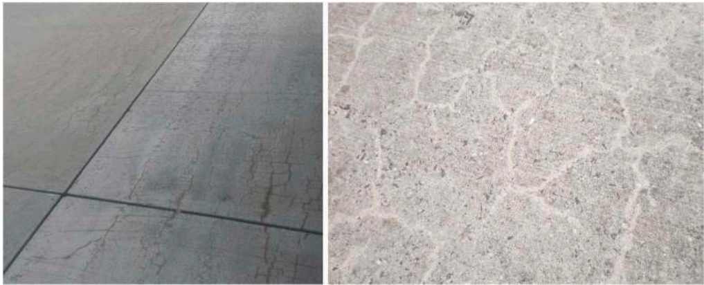
Figure 1. Examples of different types of material destruction of concrete structure.
