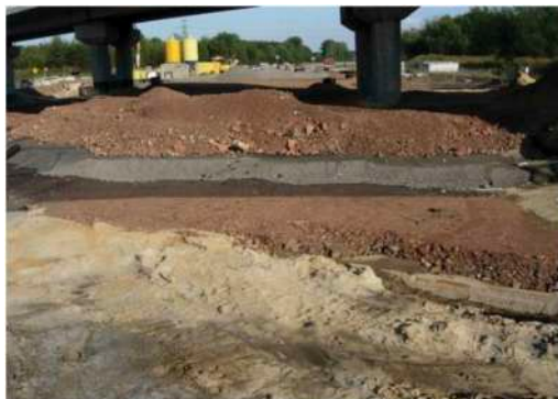
Figure 8. Example of geomattress with two layers of burnt coal mining shales (red colour) under motorway pavement - A1 motorway project in Zabrze.
