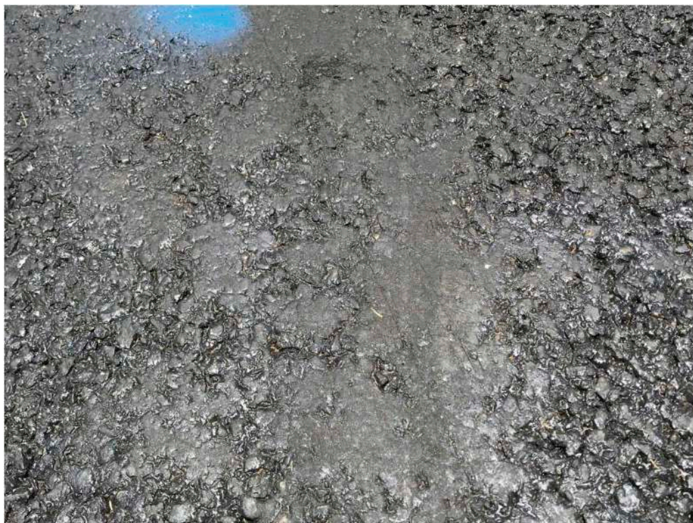
Figure 9. Example of isolated bitumen-rich area of SMA.
