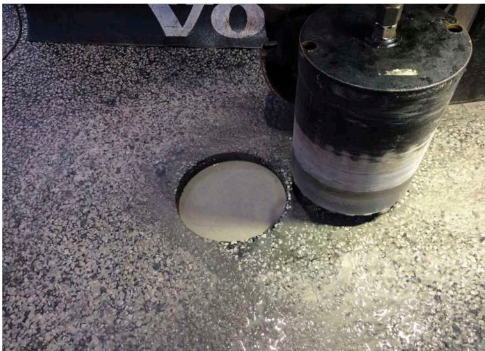
Figure 4. After drilling the cooling water did not drain through the unbound base.
