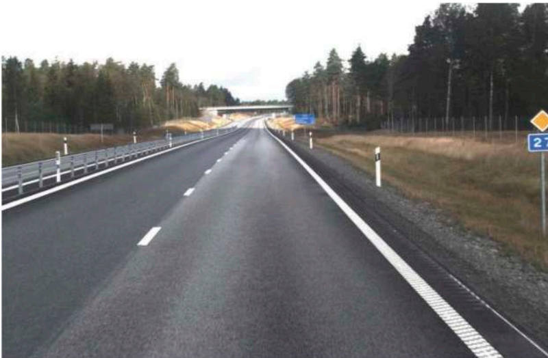
Figure 2. Photo from 2014, where samples were taken in 2019. Courtesy of STA survey.
