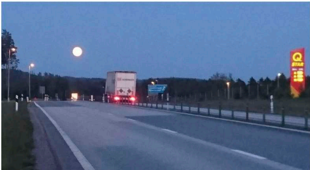
Figure 3. Coring the pavement took place one night in June 2019. Note repaired areas.
