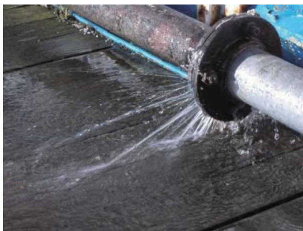
Figure 1. Pipe burst due to the high coefficient of volumetric expansion.
