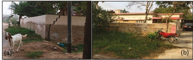
Figure 10. Signs of ground displacements in the study area. (a) Cracks in the building walls due to differential ground displacement; (b) elevation of a residential house in the University of Karachi's Professors colony has dropped to ~2 m below its base-level due to soil liquefaction caused by seawater intrusion. During the field visit, signs of soil salinity were observed in different parts of the University of Karachi.
