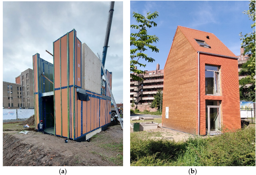
Figure 2. Living Lab Ghent (a) during construction and (b) final stage in commissioning.
